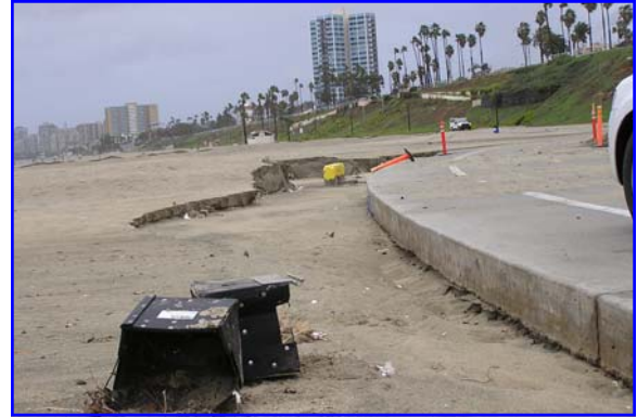
Erosion Along Bike Path
